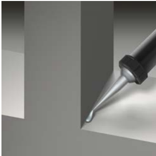
Figure 1: Apply a 10 mm diameter bead of SP525 to bottom corners of the window opening to match joint depth of tape
